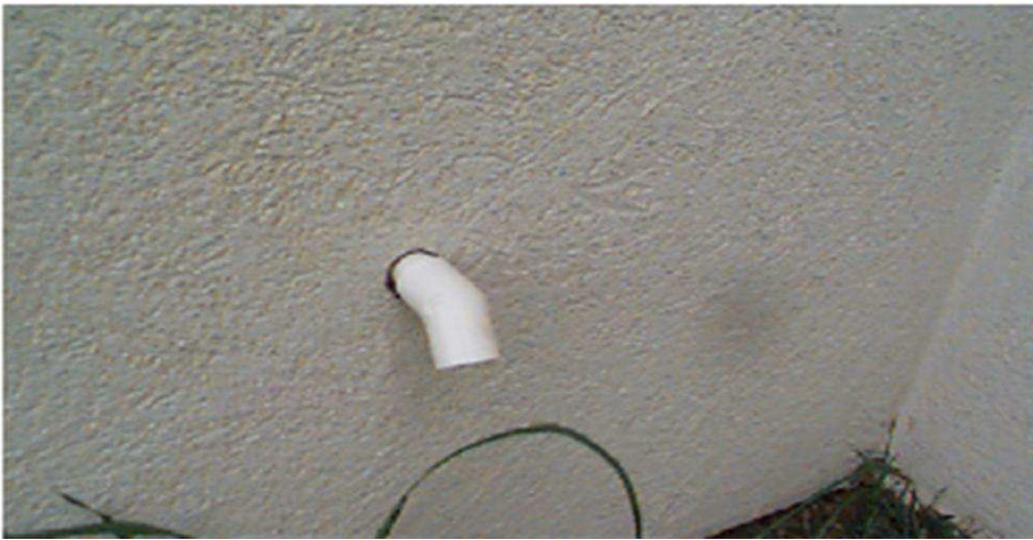
Unsealed Pipe Penetration
