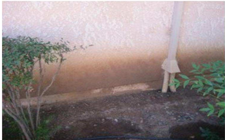
Water Splashing from Eaves
