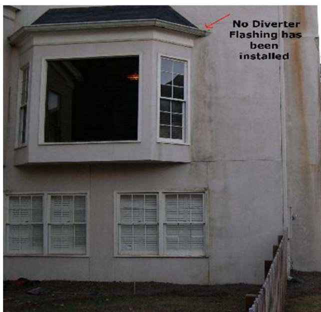
No Diverter Flashing Has Been Installed
