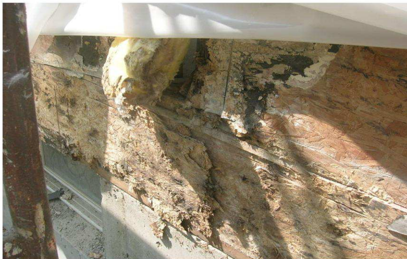
The most extensive damage is usually found below windows
