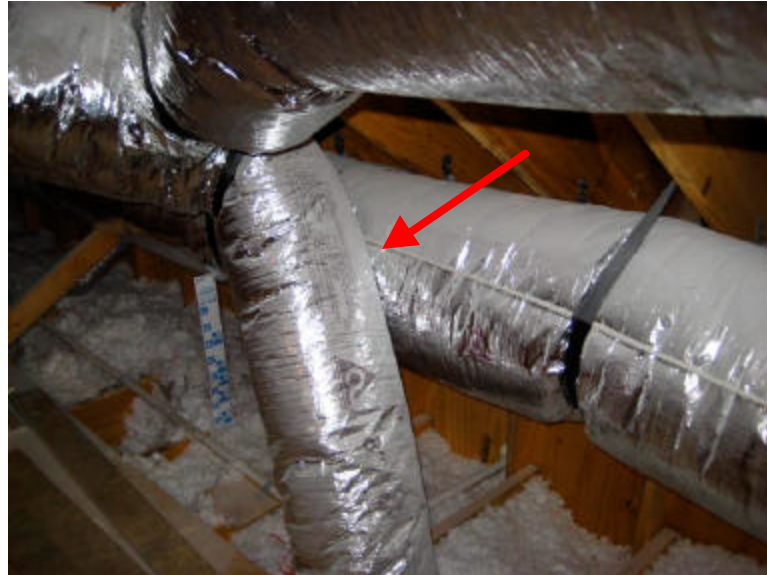
Return air filters are dirty.
